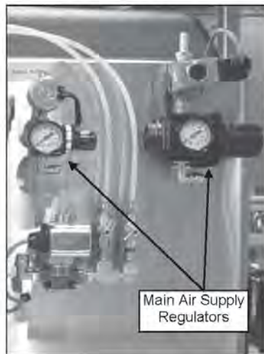
Figure 6-24. Air Regulators on pump panel
