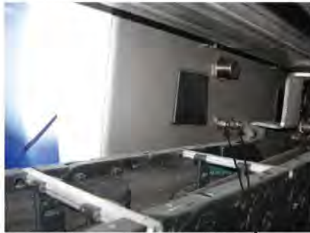
Figure 6-8. Trolley belt tensioning bolts
